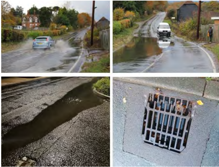
Images show examples of excess water on the roads due to blocked drains and lack of drain capacity
