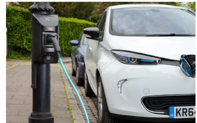
Figure 53: Example of on-street electric vehicle charging points.
