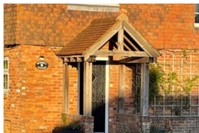
Figure 30: Timber gabled open porch with clay tile roof over low brick walls
