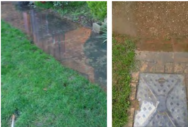
Images show sewage surcharge as a result of heavy rainfall
