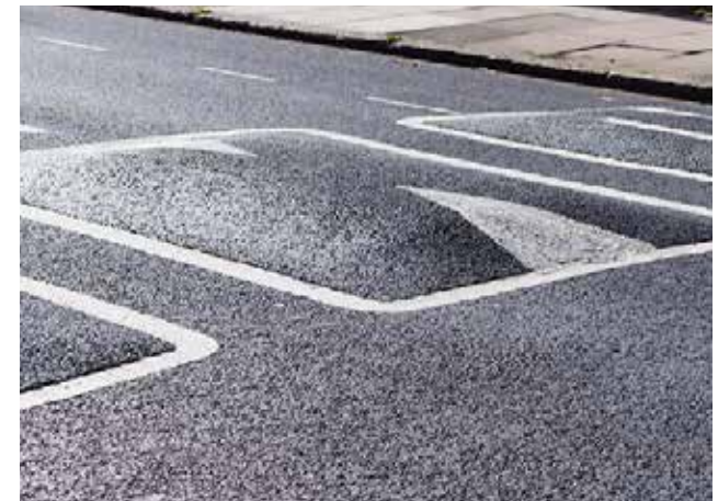
Figure 54: Example of a speed cushion.
