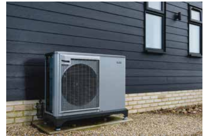
Figure 106: Example of an electric heat pump that is placed to the back of the house, whilst its grey colour fits nicely with the black weatherboarding of the property.
