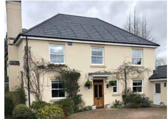
Figure 107: Use of shingle-like solar panels on a slate roof, with the design and colour of the solar panels matching those of the adjacent slate tiles.
