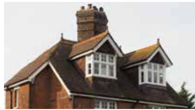
Hipped roof with Kentish peg tiles and details such as ornamentation of chimney, ridge line and timber work
